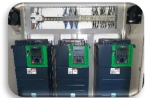
Inverter Installation for machineries
