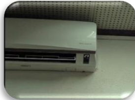
Inverter AC Installation
