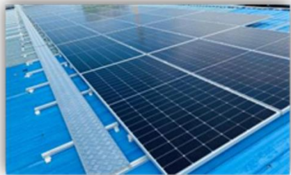
1 MW Solar system installation at GLTP Kandy connected to grid
