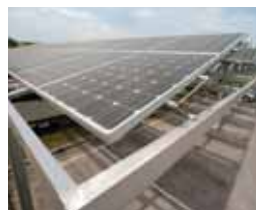
Solar Powered PMD Ventilation System
